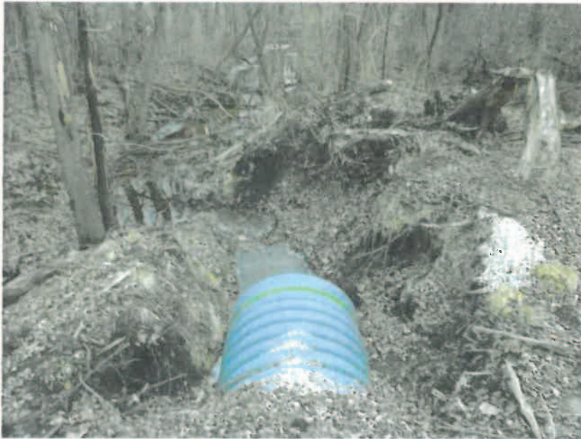
Figure 12 Owners of Vacant Lots Must Remove Branches and Maintain a Flow Path to the Dutch Gap Canal.
